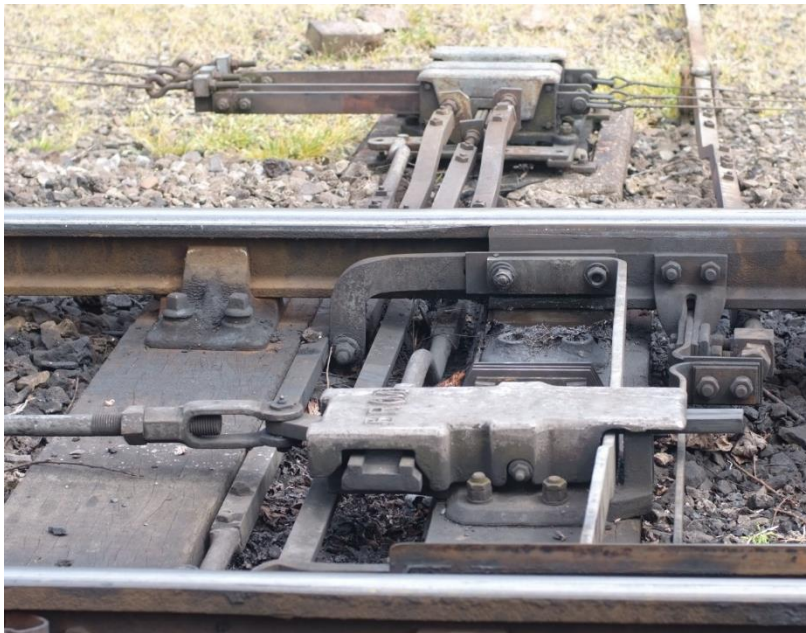
6 A closer view of a point with facing lock and signal detection, quite close to the point
